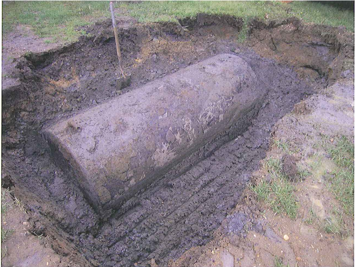
UHOT ready to be removed, note wet soil around UHOT (in this case it is an oil/water mix)
