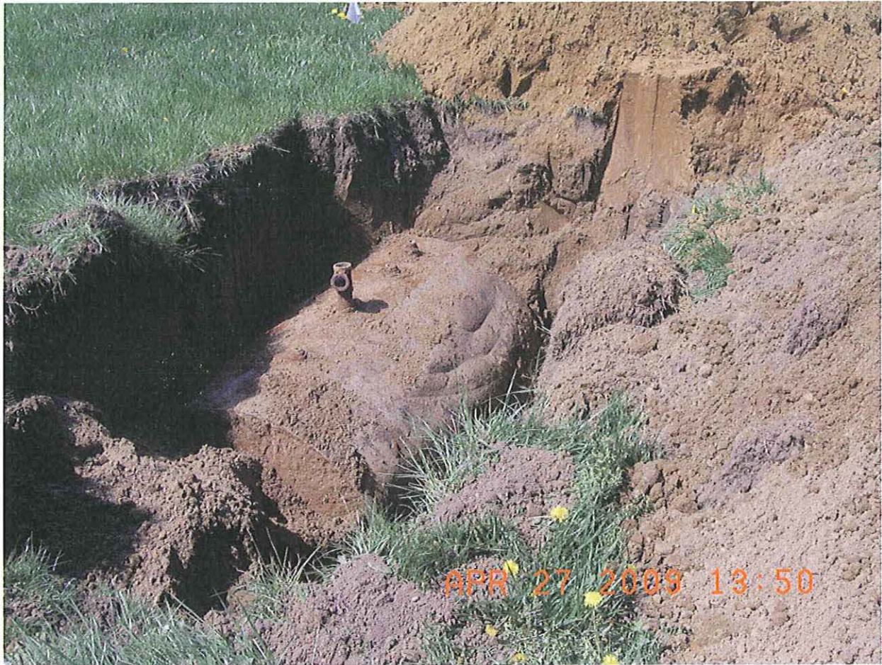
Top tank exposed, note no piping found at tank
