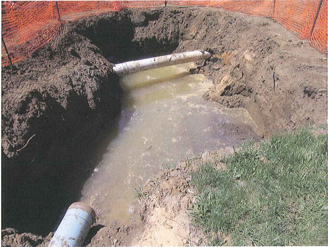
Pipe run at 538
