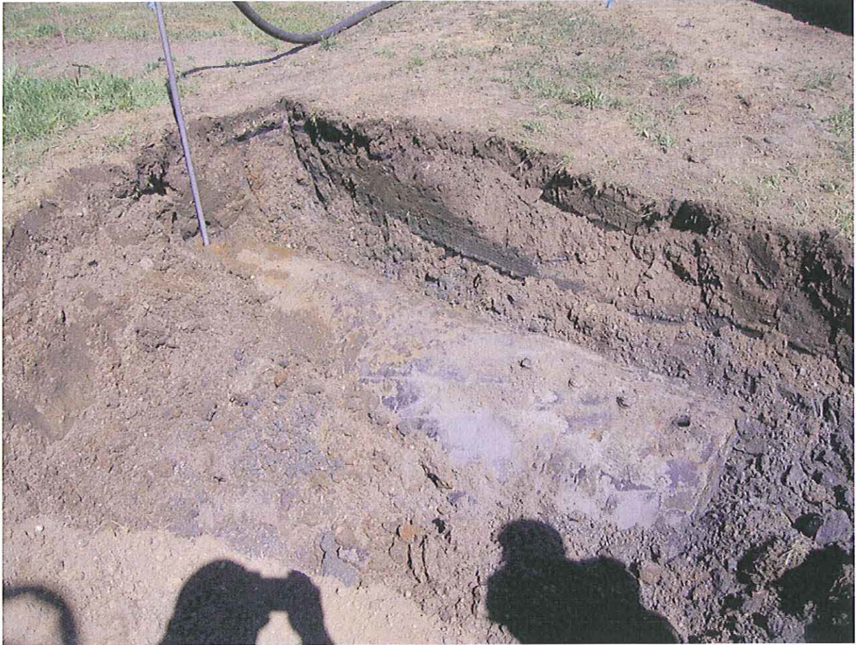
Top of UHOT at 541, removing product from UHOT before removal
