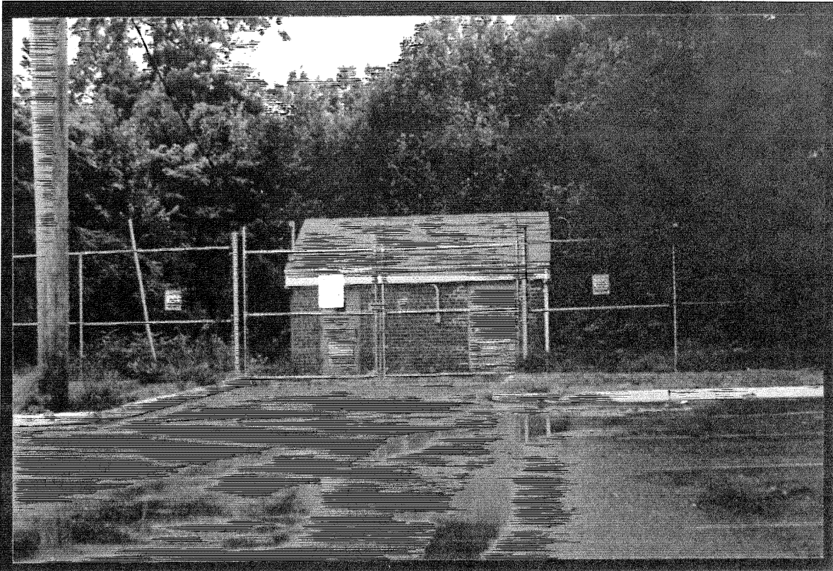
Sewage Pumping Station (CW-8)
