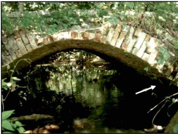
Figure 4-12. Site 28MO385, Brick Culvert, View North Showing Present Conditions, Including Missing Brick on Intrados (arrow)
