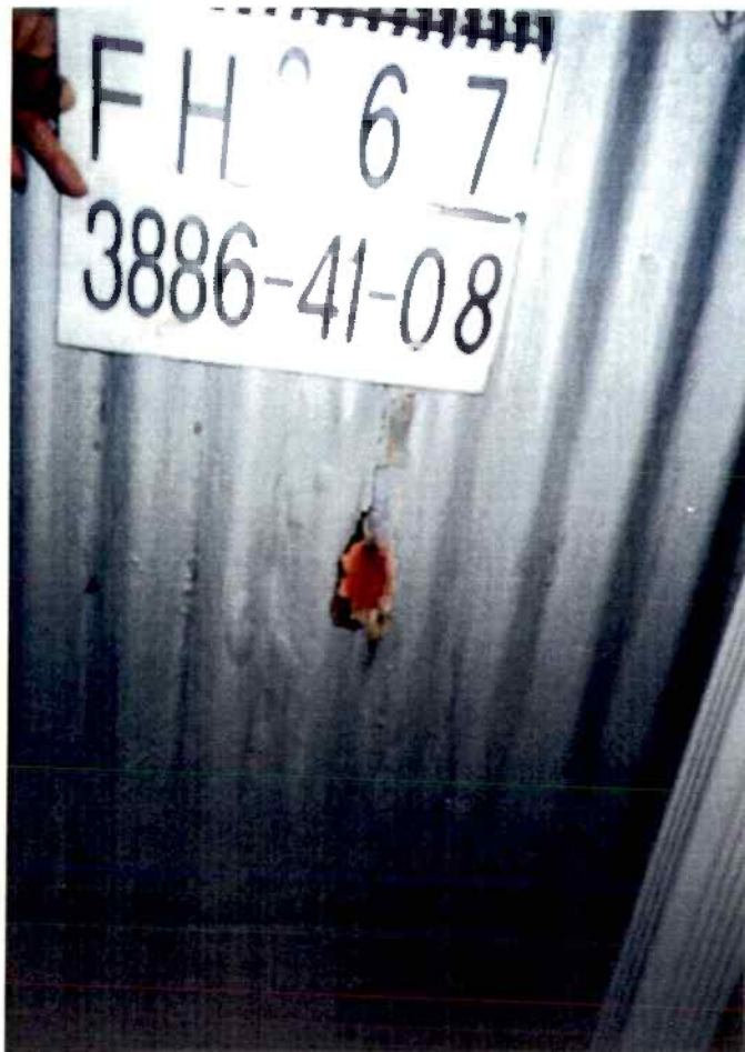
EXTERIOR WALL: (SAMPLE FH867) BROWN EXTERIOR BUILDING PAPER TESTED POSITIVE.
