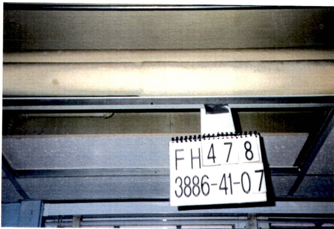
Bldg. 2525 Room 2101: Sample FH478, 4 - 8" pipe run tested positive; sample FH480 (not shown) 4 - 8" pipe run also tested positive.
