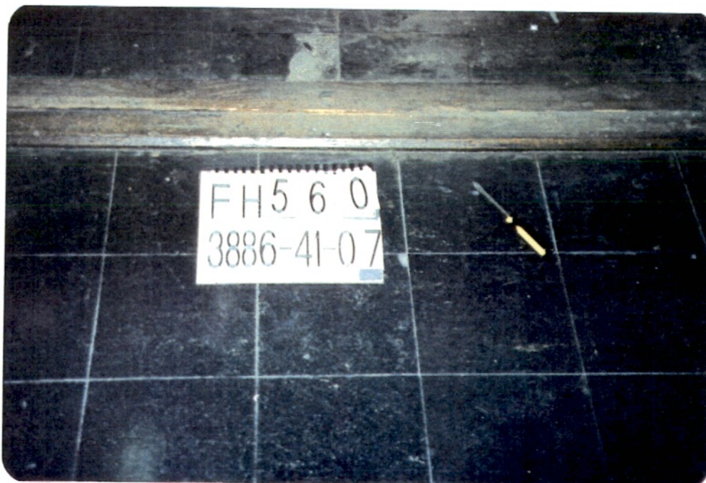
Bldg. 9011A - Mechanical Room: 9 x 9" black floor tiles FH560 tested positive, Office 1A; 9 x 9" black floor tiles FH559 also tested positive. Metal shop storage 9 x 9" black floor tiles FH558 also tested positive.
