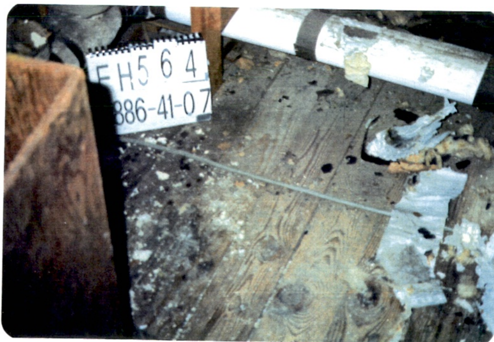
Bldg. 9011A - Attic Area: 4 - 8" mud fitting sample FH564 tested positive.
