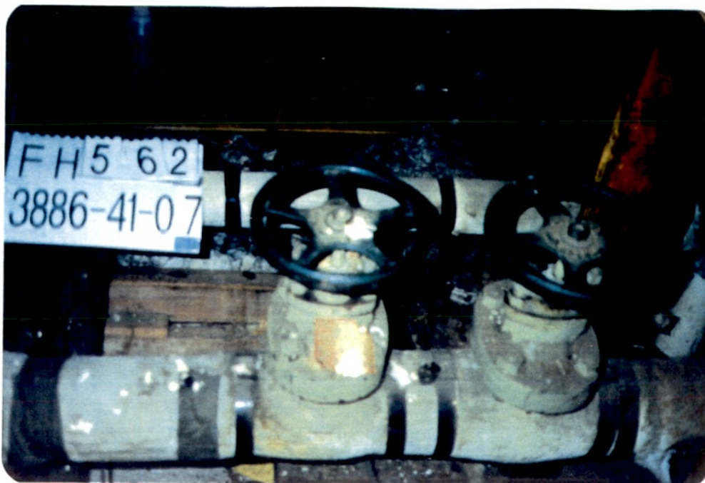
Bldg. 9011A - Attic Area: < 4" steam fitting FH562 tested positive. Sample FH563 < 4" pipe run (not shown) also tested positive.
