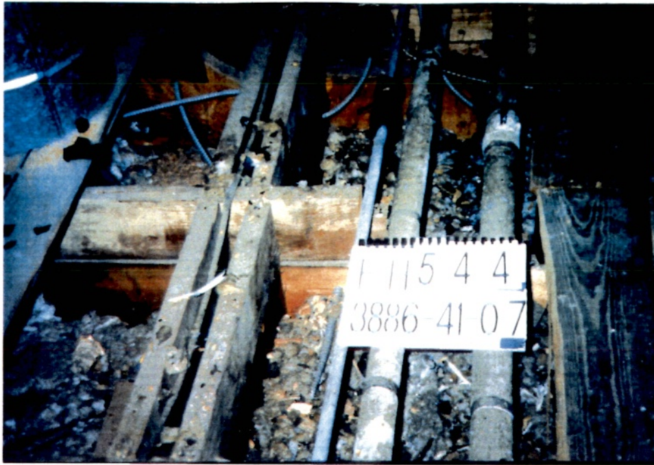
Bldg. 9011D - Attic: < 4" pipe run sample FH544 tested positive, also testing positive and not shown are samples FH546 4 - 8" pipe run; sample FH548 < 4" pipe run; sample FH550 4 - 8" pipe run.
