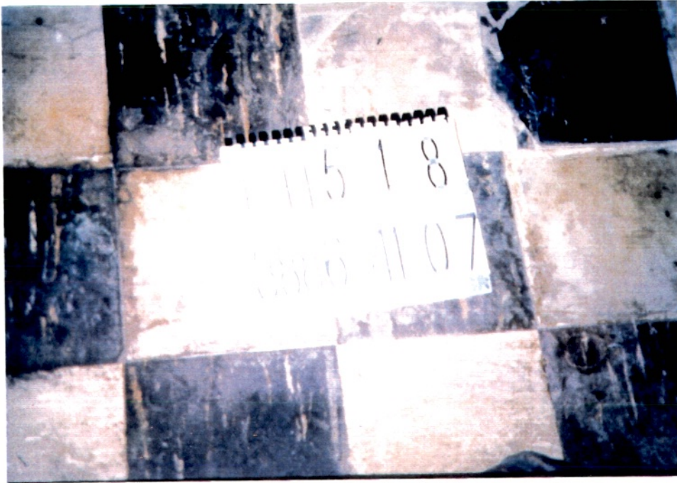
Bldg. 2704 - Test Chamber, Mechanical Room: 9 x 9" floor tiles tested positive. Samples FH516; FH517; FH519 and FH520, floor tiles (not shown) all tested positive.
