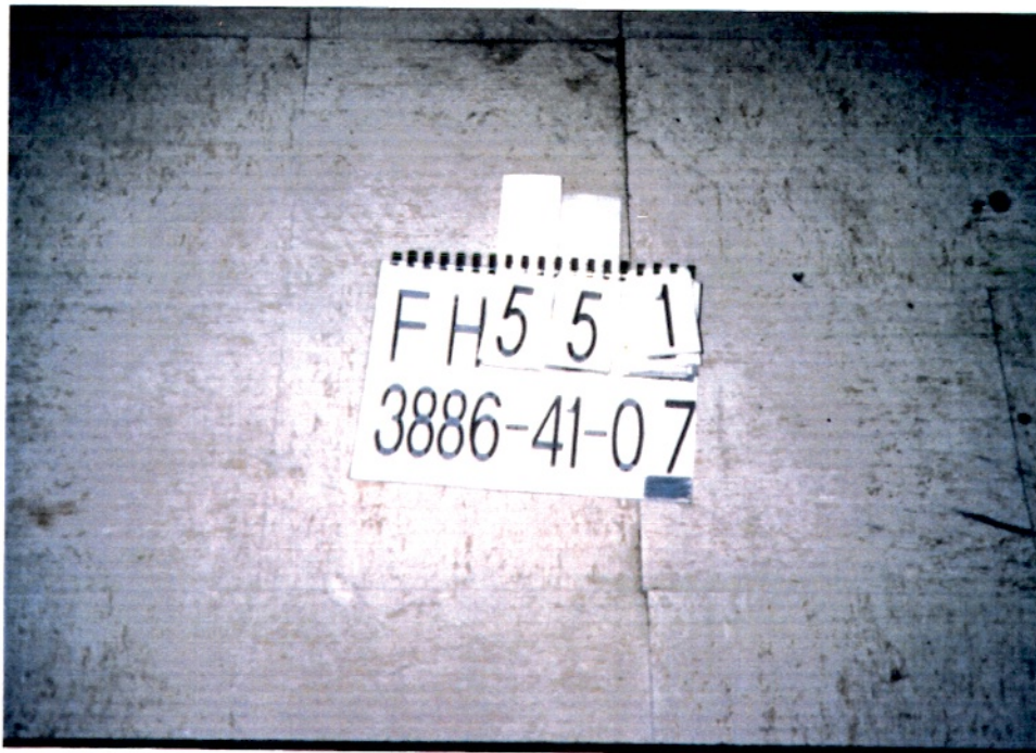
Bldg. 9011D - Corridor D: Sample FH551 12 x 12" tan floor tiles tested positive; sample FH552 (not shown) 9 x 9" red floor tiles also tested positive. Following floor tile samples tested positive (not shown) are: FH557, 12 x 12" tan; FH558, 9 x 9" black, FH559 and FH560 also 9 x 9" black.
