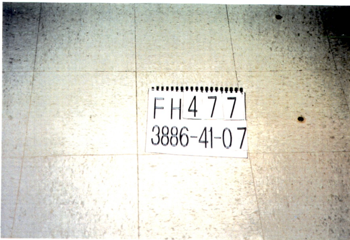
Bldg. 2525 Room 2101: Sample FH477, 12 x 12" tan floor tiles tested positive.
