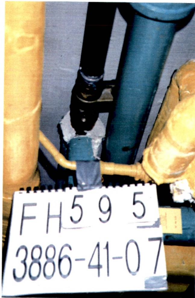
Bldg. 9042 - Basement: Sample FH595 < 4" mud fitting tested positive.
