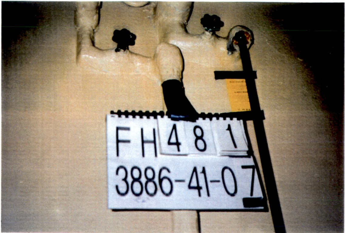
Bldg. 2525 Room 2102A: Sample FH481, < 4" mud fitting tested positive.
