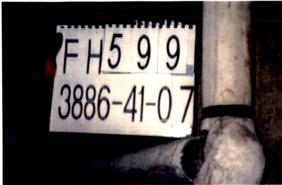
Bldg. 9042 - Basement, Corridor leading to Pipe Tunnel: Sample FH599 < 4" mud fitting tested positive; sample FH600 < 4" pipe insulation also tested positive.
