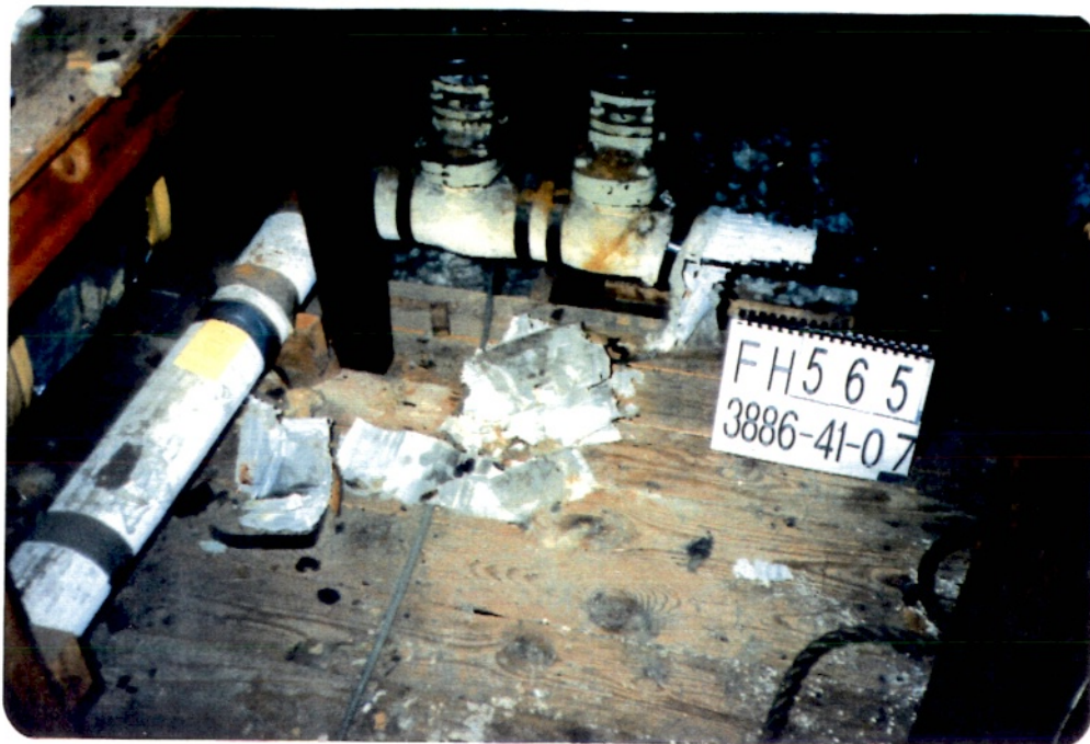
Bldg. 9011A - Attic Area: 4 - 8" steam pipe insulation sample FH565 tested positive.
