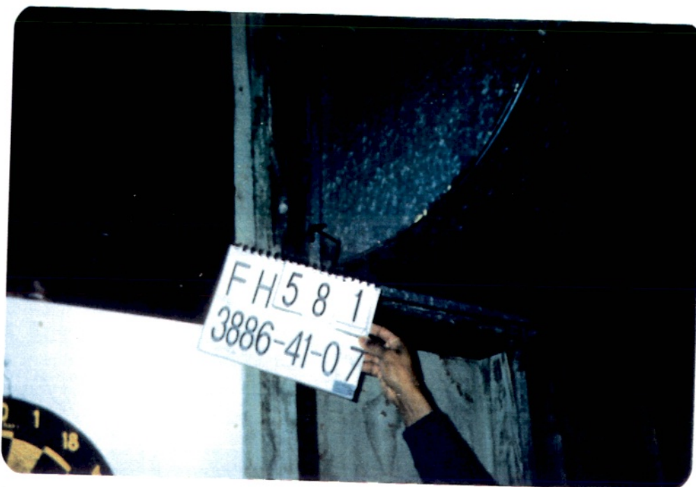
Bldg. 9009 - Serv-Air Garage/Shop: Expansion joing around metal duct, sample FH581 tested positive.
