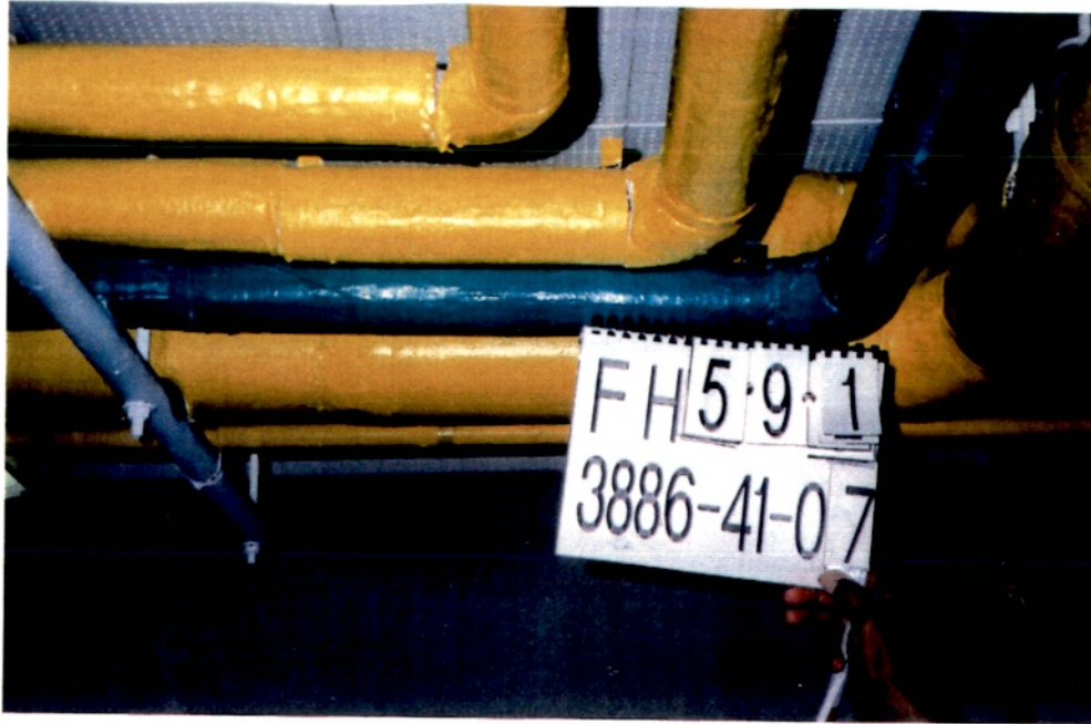
Bldg. 9042 - Basement: Sample FH591 < 4" mud fitting tested positive. Samples FH592 < 4" pipe run; sample FH593, 4 - 8" mud fitting; and sample FH594, 4 - 8" pipe run all tested positive.
