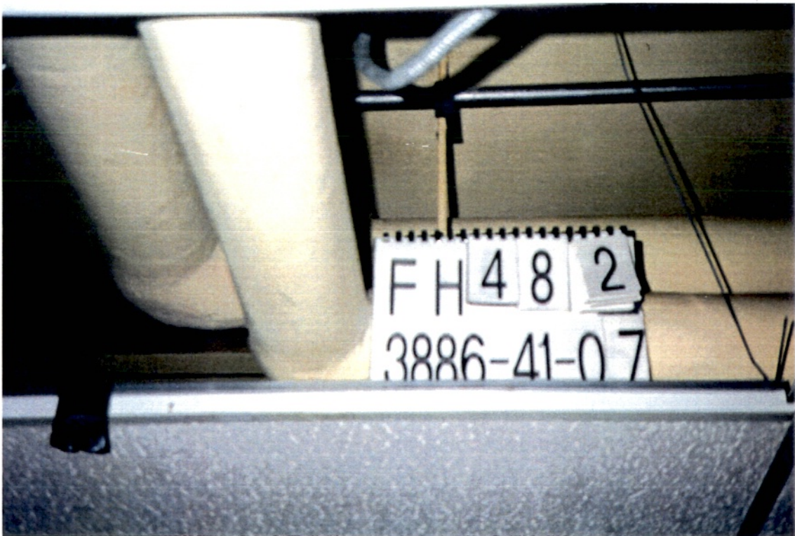
Bldg. 2525 Room 2105A: Sample FH482, 4 - 8" mud fitting tested positive. Samples FH484 (not shown) 4 - 8" mud fitting tested positive.
