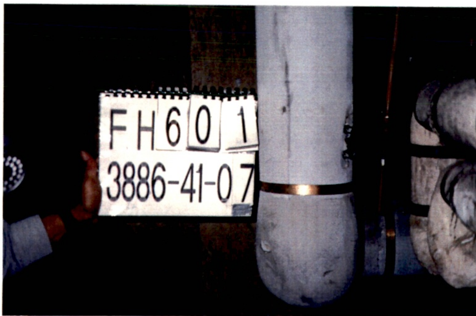
Bldg. 9042 - Basement, Corridor leading to Pipe Tunnel: Sample FH601, 4 - 8" mud fitting tested positive. Sample FH602 (not shown), 4 - 8" pipe run also tested positive.
