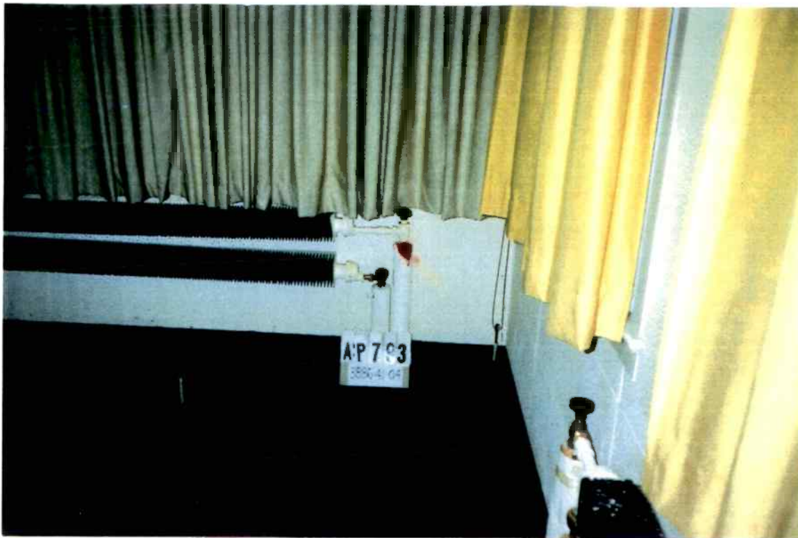
AP793 - Rooms 202, 202B, and 202C - Pipe insulation tested positive for asbestos.
