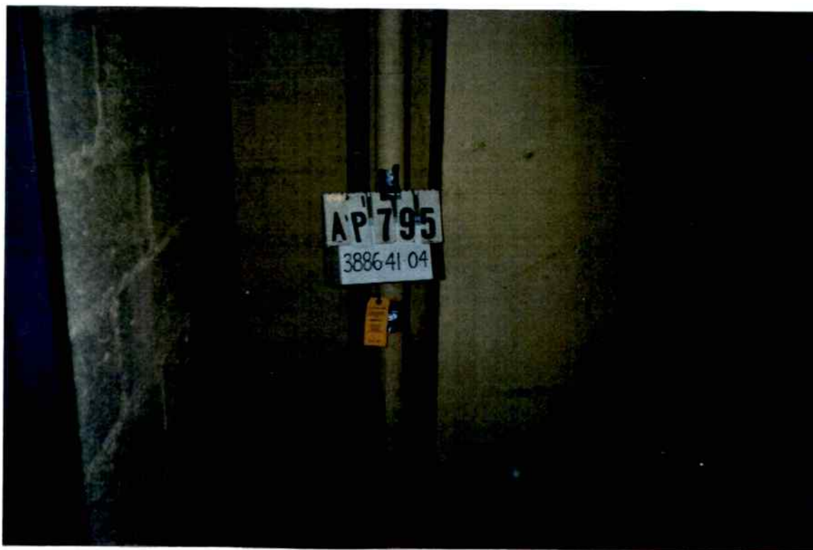
AP795 - First Floor Closet - Pipe insulation tested positive for asbestos.
