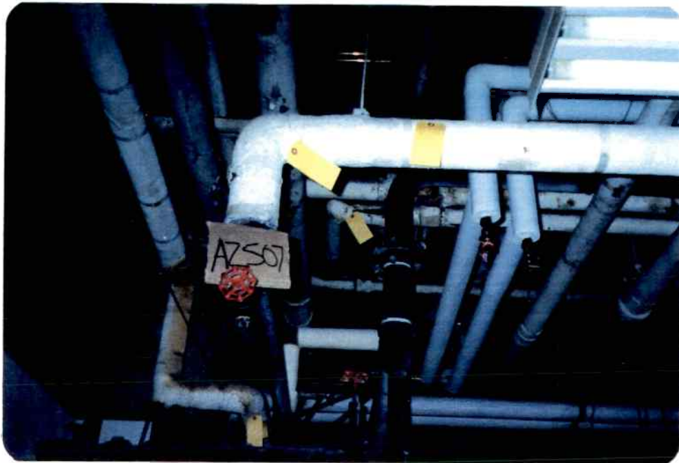
AZ507 - Bldg. 1075 (Hospital) Boiler Room 4-8" pipe fitting tested positive for asbestos.
