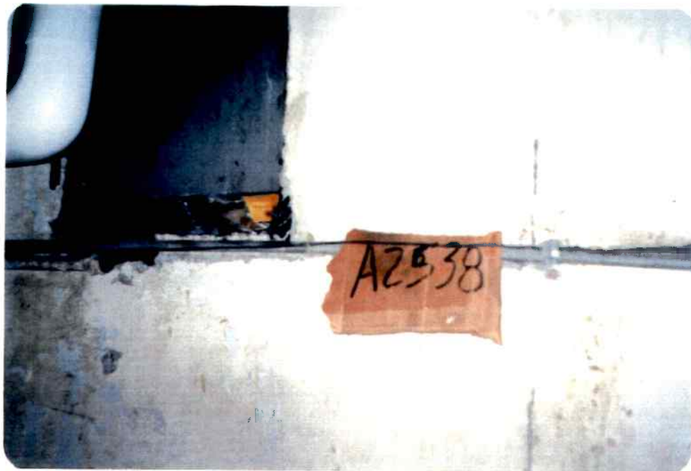
AZ538 - Boiler Room - Air handling equipment insulation tested positive for asbestos.
