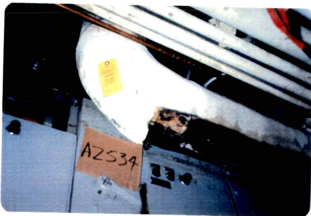
AZ534 - Boiler Room 9-14" pipe fitting tested positive for asbestos.
