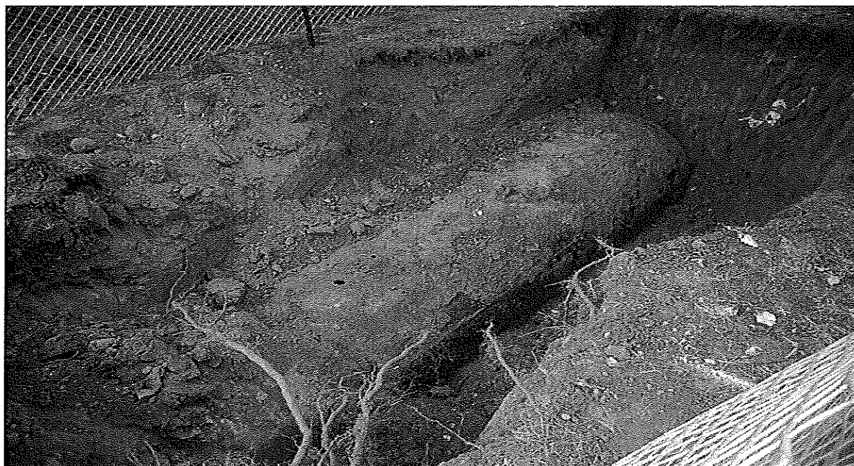
UHOT at Bldg. 1123
