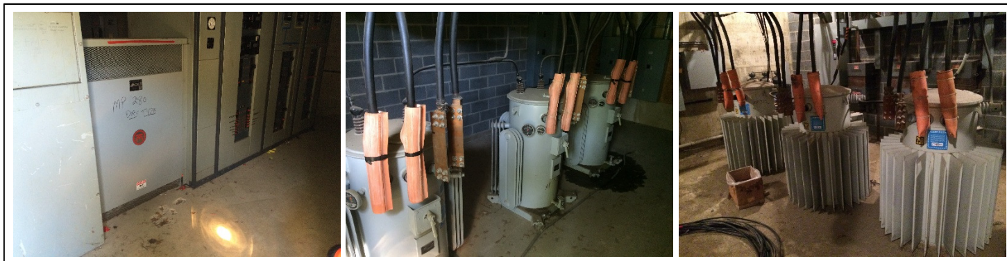
Figure 2 – Former Electrical Transformers at Buildings 1002 (left), 1208 (center), and 1209 (right).
